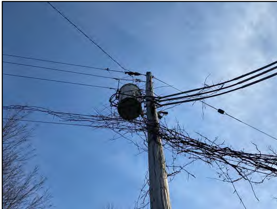
Photo 6. Transformer on subject property Photo facing east
