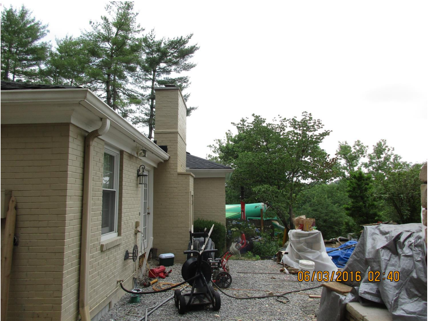
Looking at the rear of the property where the roof would continue for approximately 36.5' ft.
