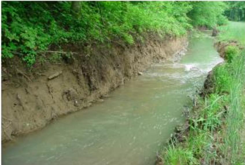
Below: Stream with degraded habitat, severe erosion causing downstream pollution.
