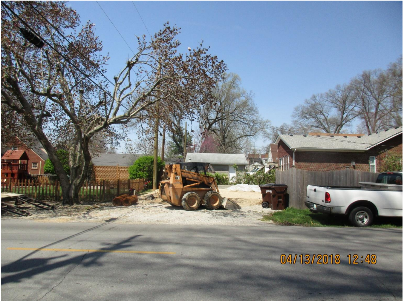
The location of the requested variance and the driveway to be replaced with concrete.
