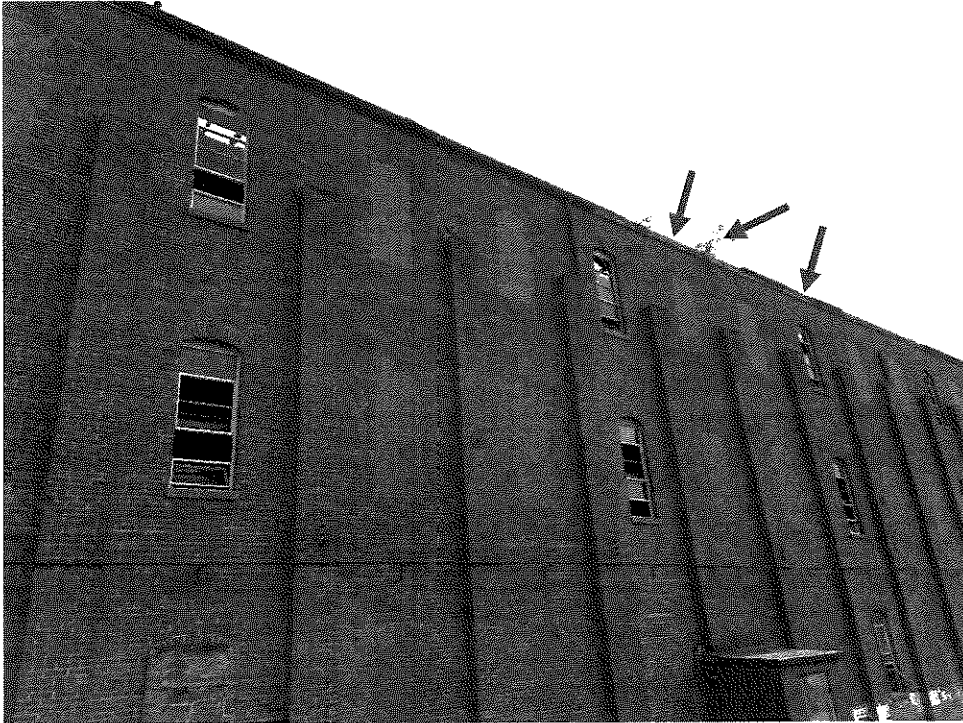
Photo 3 - South side of building. Large plant growth is visible. Missing gutters from deteriorated roof framing. White spots in upper windows are areas where the roof has collapsed.
