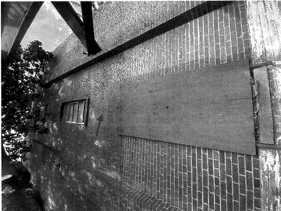
Photo 8 - East side of the northeast corner of the building. Cracks extending up the height of the wall and loose bricks over the lower arch top window.
