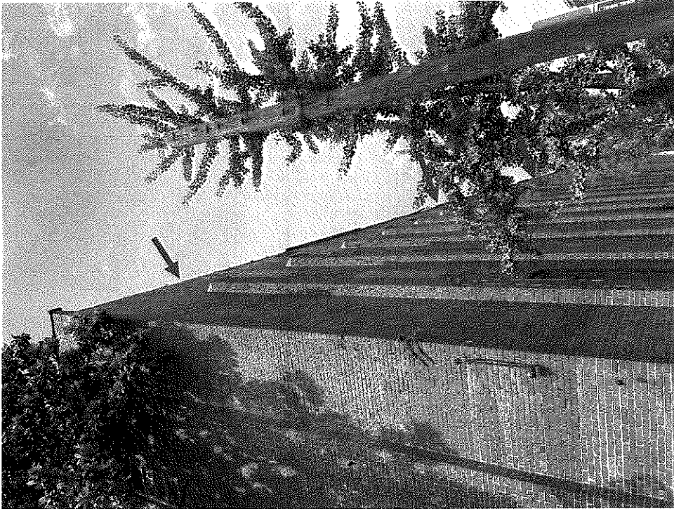
Photo 9 – Northeast corner of the building. Missing gutters along most of the length of this wall due to deteriorated roof framing.
