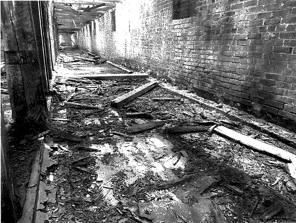
Photo 21 – Debris from collapsed framing on the floor and has broken a framing member at the next level up. Base of column is severely deteriorated.
