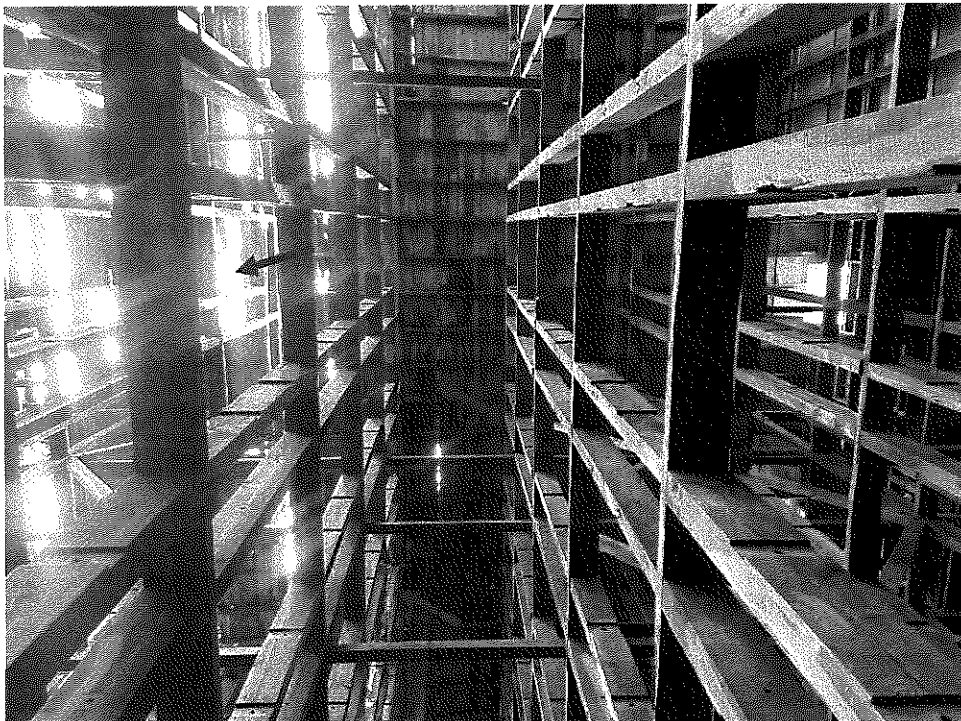
Photo 22 – Large area of collapsed roof. Deteriorated column in upper level of wood framing with severe mold growth. A better section of the visible roof with severe water damage. No 4x4 dunnage framing is visible; therefore, the posts are laterally unstable side-to-side.
