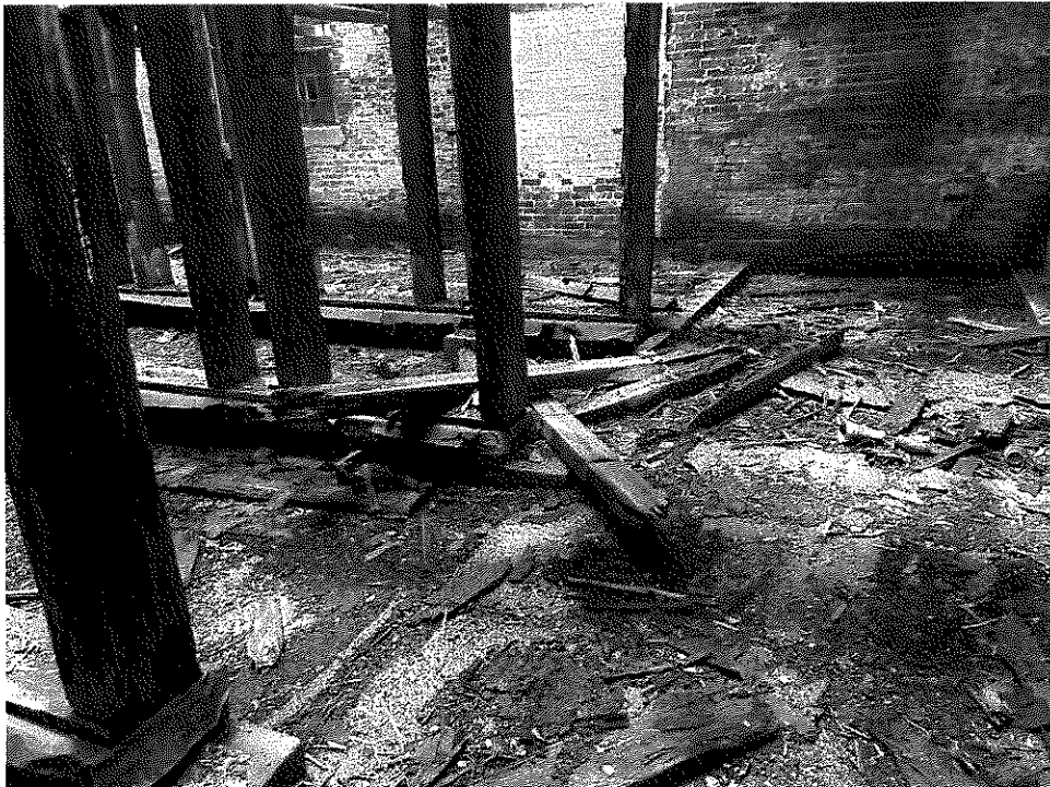
Photo 18 – More debris from collapsed roof. Most of the light in this area is from the collapsed roof.
