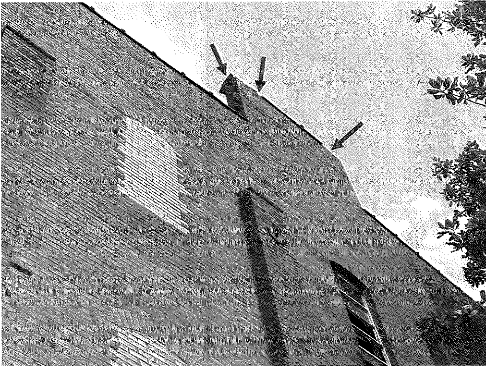
Photo 7 – East wall cap is missing and dislodged.
