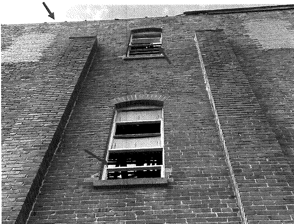
Photo 10 – North wall of the building. Missing gutters along most of the length of this wall due to deteriorated roof framing. Blue color in windows is collapsed sections of roof.
