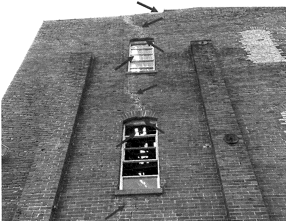
Photo 12 – West side of the northwest corner of the building. Missing cap at top of wall, cracks in old pointing repairs, and bricks in the arch tops of the windows about to fall. White spots seen in the windows are areas of collapsed roof.
