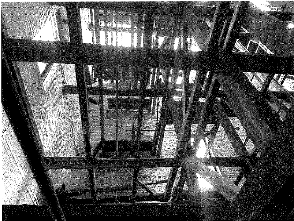
Photo 14 – Interior wood framing with deteriorated and molded wood. Large area of collapsed roof is visible.
