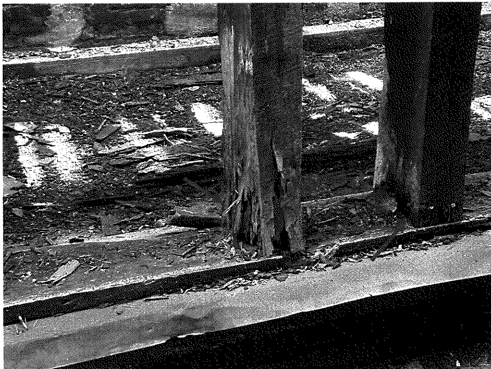
Photo 16 – More deteriorated column bases. Nails from the toenail connection is visible in the right column. They are becoming exposed due to deterioration of the wood material.
