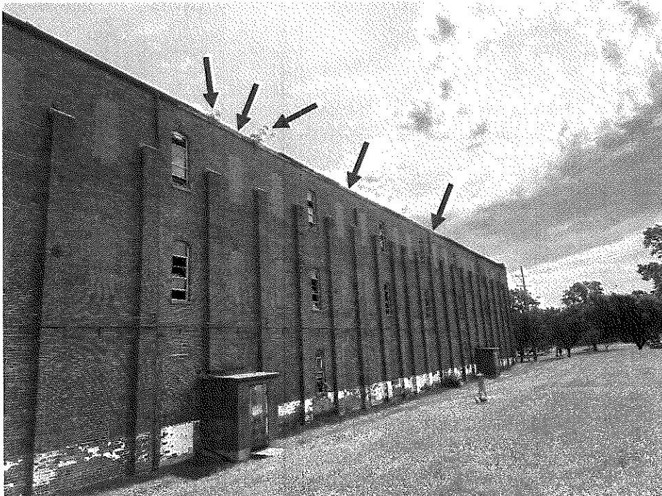
Photo 2 - South wall of the building. Large plant growth is visible. Missing gutters from deteriorated roof framing.
