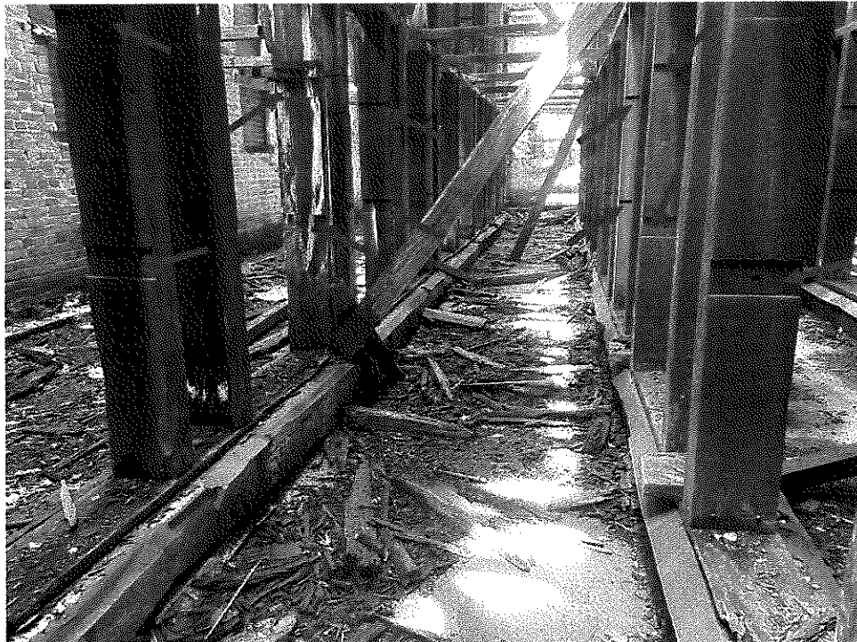
Photo 20 – Collapsed framing and debris from collapsed roof. Missing dunnage locations are easily visible. Third column on left has severe mold growth.
