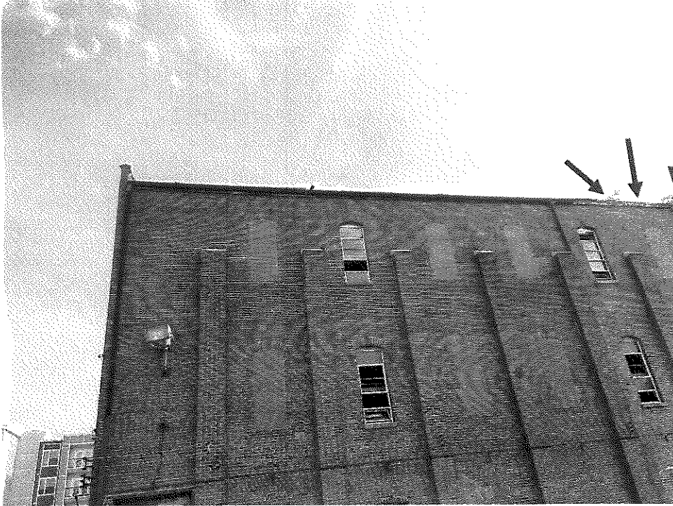
Photo 1 - South side of the southwest corner. Large plant growth is visible. Missing gutters from deteriorated roof framing.
