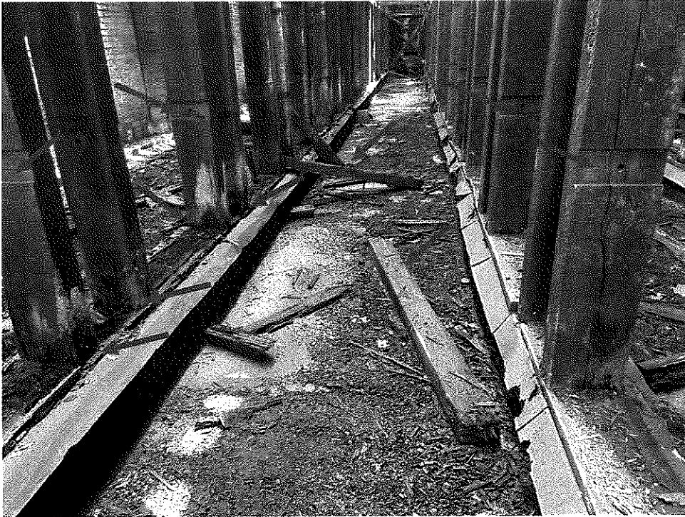
Photo 17 – Deteriorated post bases and debris from collapsed roof above. The notches in the posts with the hole in them are the locations where the 4x4 dunnage should be.
