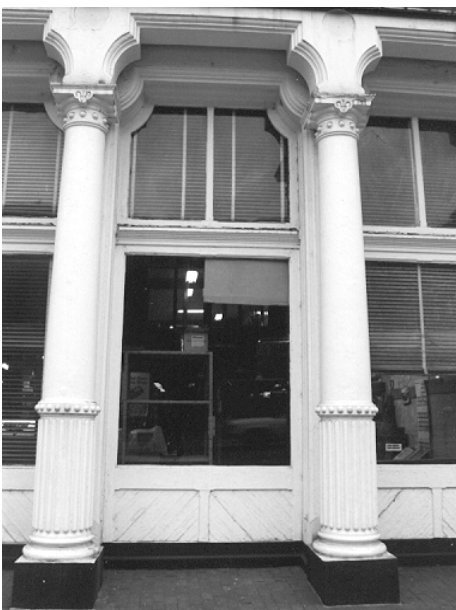
Clean hard metals, such as these cast-iron piers, to remove corrosion and paint build-up. Low-pressure grit blasting may be used only if additional cleaning is required.
