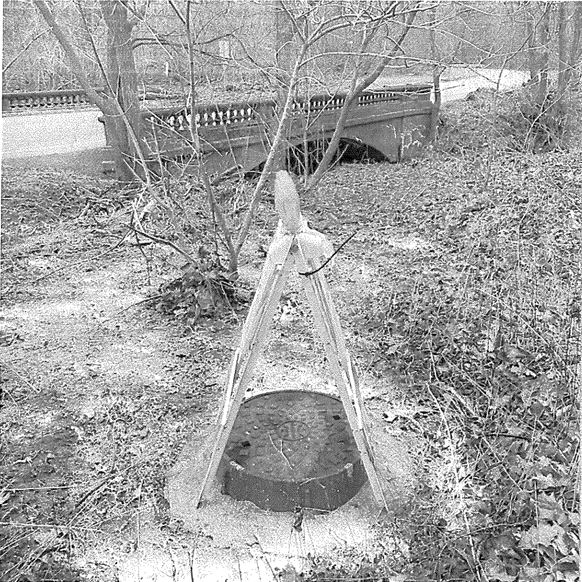
Photo: Sewer Overflow location Cherokee Park January 8, 2023 with MSD warning and lime spread on ground.
