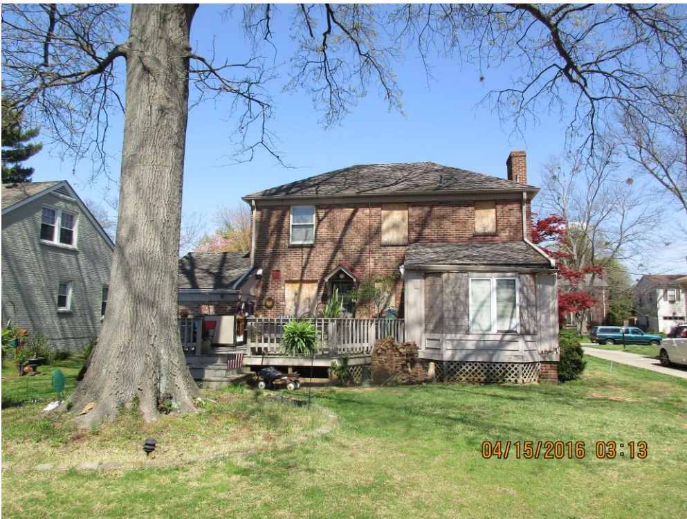
Looking at the rear of the property where the proposed addition is to be constructed.
