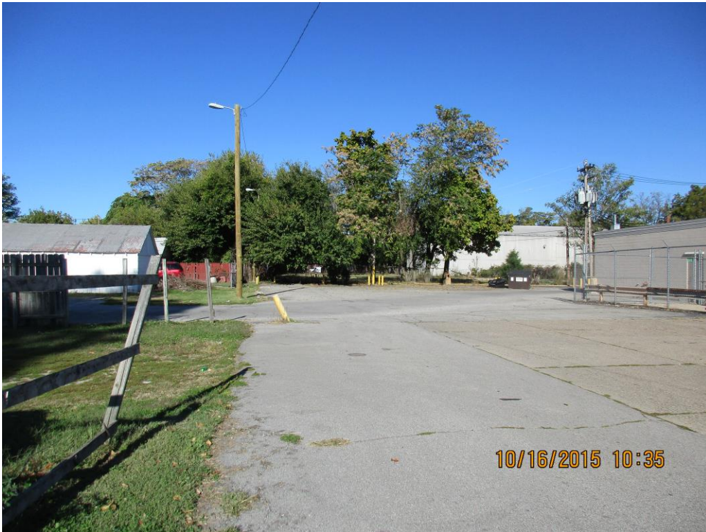
Location of the parking encroaching into the rear landscape buffer areas (LBA)
