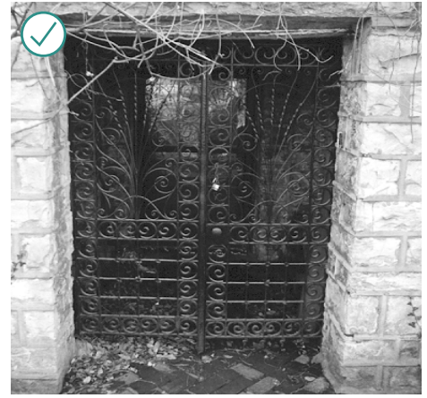
Install security bars of simple design that do not obscure the architectural character of the original doors or damage historic fabric. Here, a historic metalwork door secures an Old Louisville entrance.
