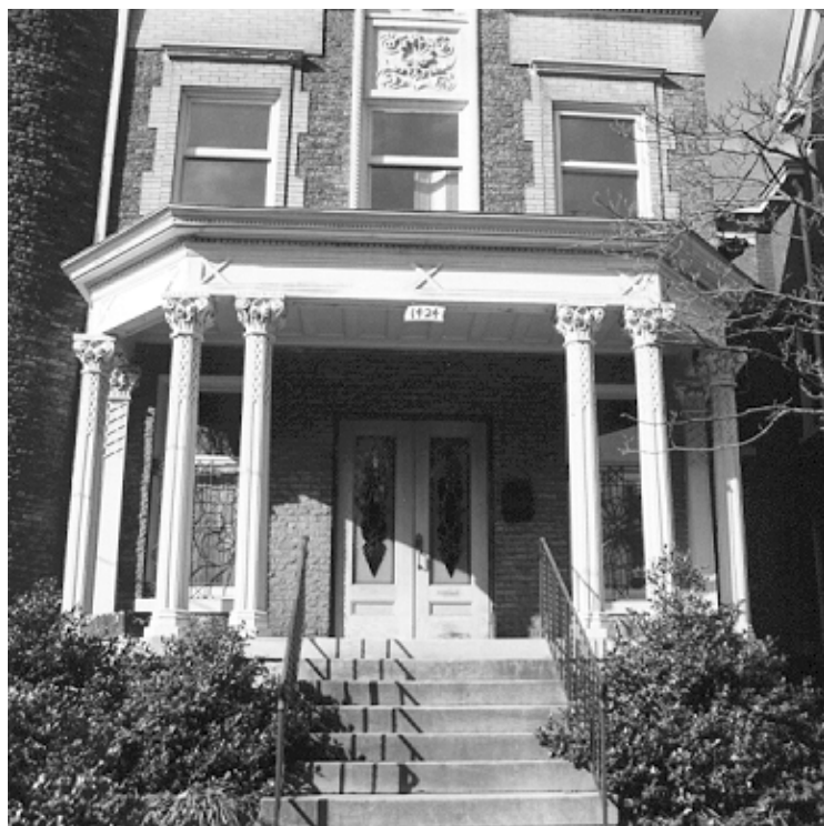
Top Right—Even if a porch replacement were appropriate, the materials used were not. Top Left—Porches were designed for many historic apartment buildings to allow residents to take advantage of refreshing breezes. Above—An intricately carved wood porch lends a stately air to an Old Louisville mansion.
