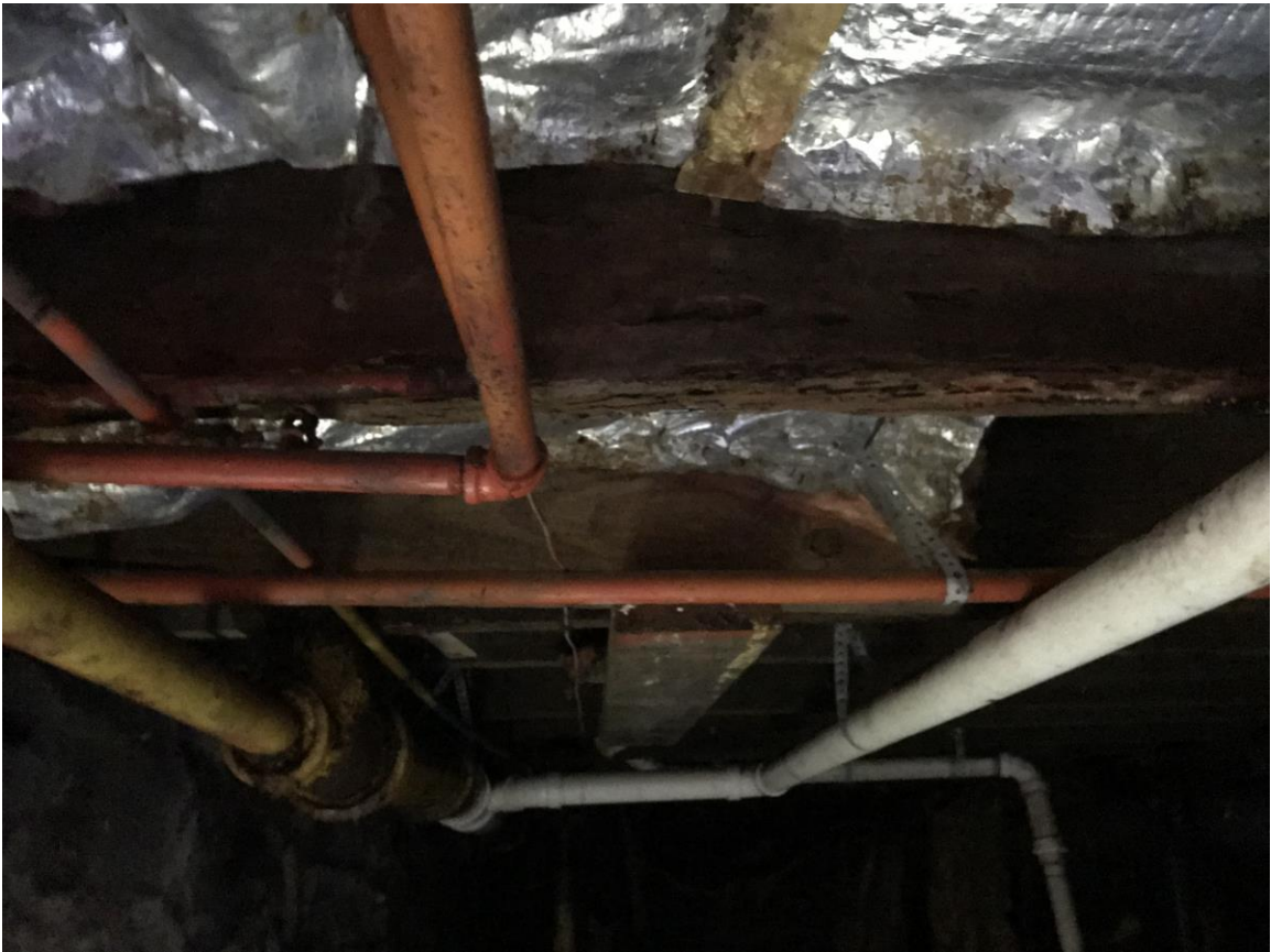
Termite damage in existing floor framing.
