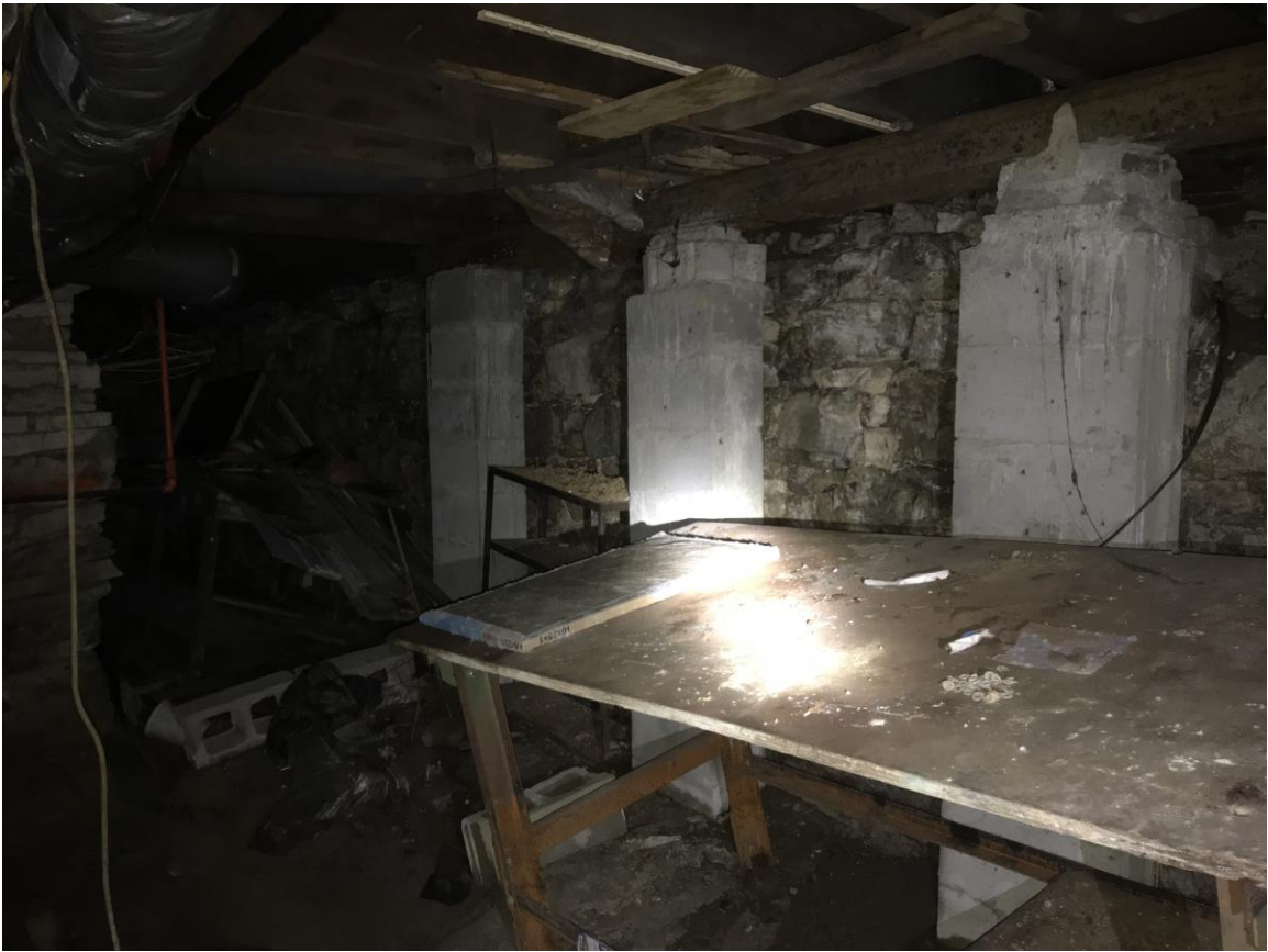
Previous repair for floor framing at basement wall.
