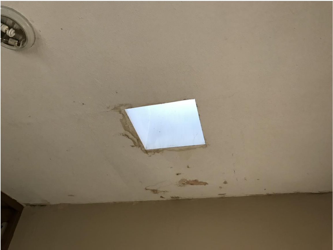
Water staining and damage to existing ceiling.
