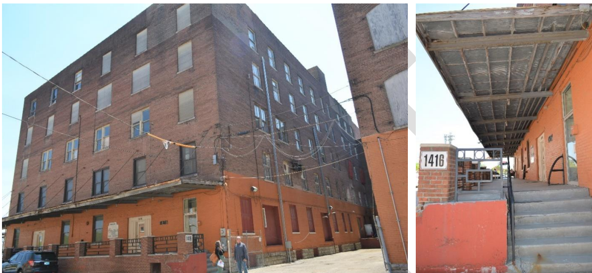
(Left) North and east facades of ca. 1911 warehouse addition; (Right) Detail of former loading dock now porch with shed-roof metal awning (J. McCarron)
