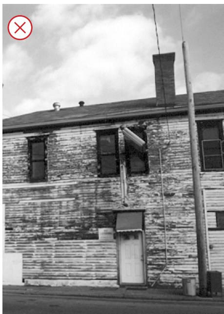
Restore the visibility of an original historic material that has been covered.
