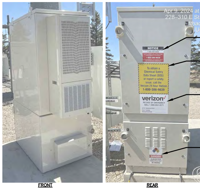
FIGURE 1 - EQUIPMENT CABINET SIGNAGE
